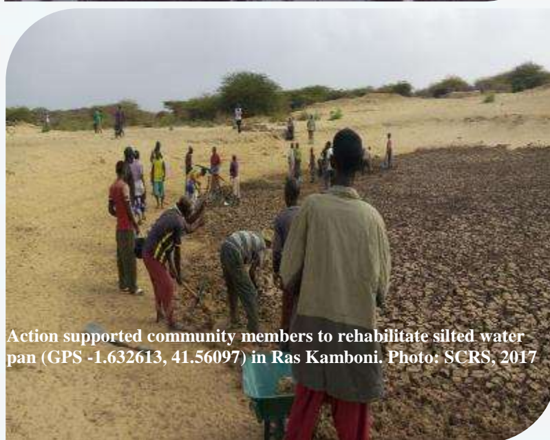
Witu community members install dam liner in a pond for RWH. Photo: Muriithi/ICRAF, 2016
