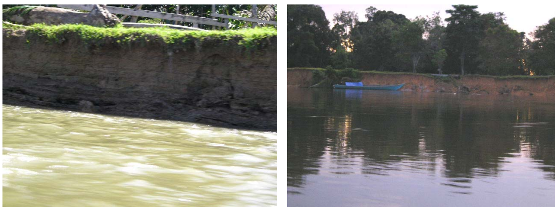
Figure 1 River bank collapse along the river in Kapuas (left) and Sibau (right)
