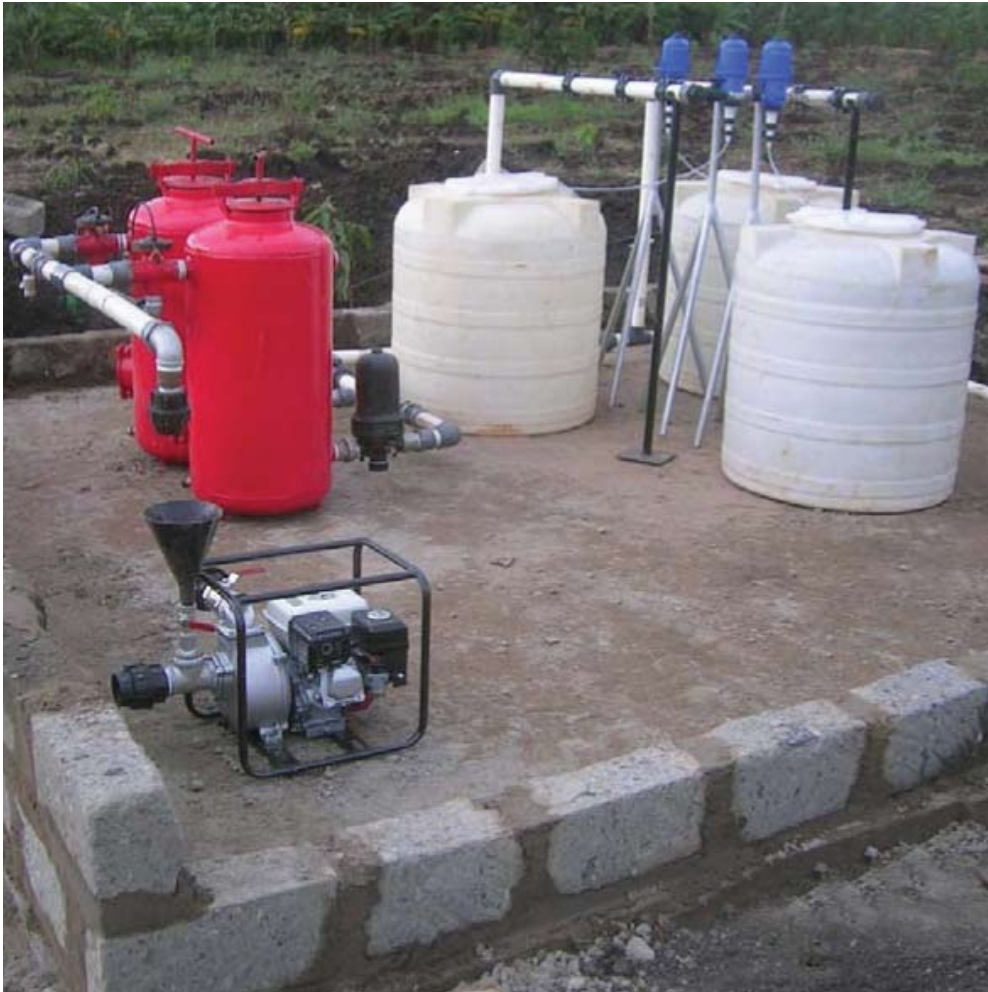
Figure 33: Pumping and fertigation equipment
